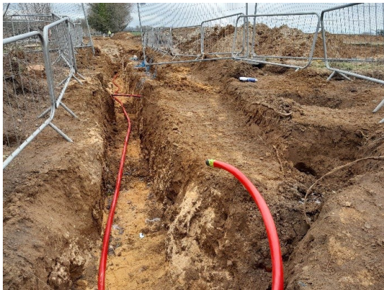
Figure 1: New HV Cable
