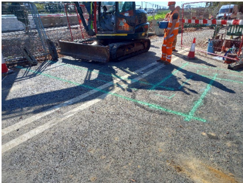
Image 1 Saw cuts in tarmac
