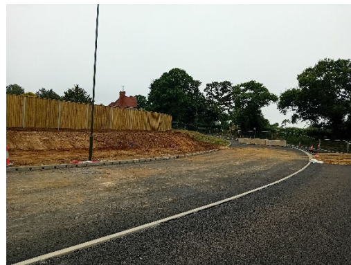
Image 5 Acoustic fencing along link road
