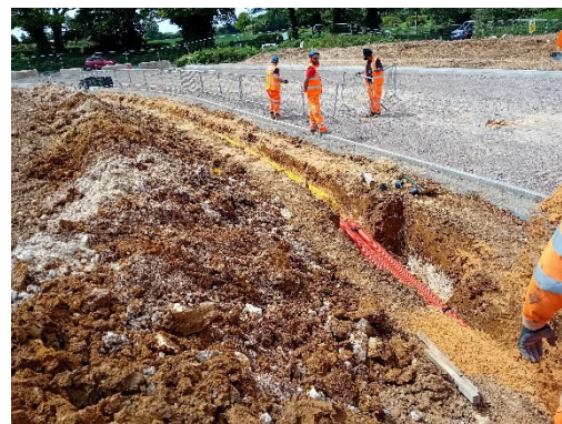
Image 5 Street lighting ducts.
