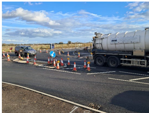
Figure 3- refuge island and white lining
