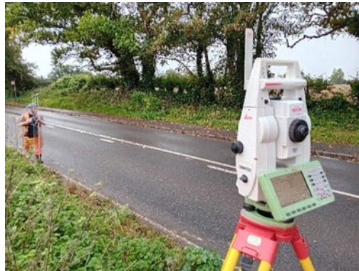
Image 3 Total station used to build up image of how bypass will connect with existing road, A284.
