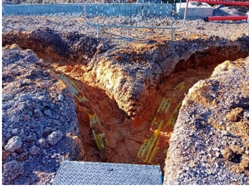
Image 3 Street lighting ducts into box.
