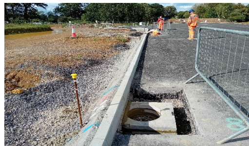
Image 2 Road gully without grating.
