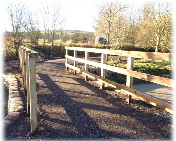
The new culvert taking for the realigned Downs Link bridleway at Bramber
