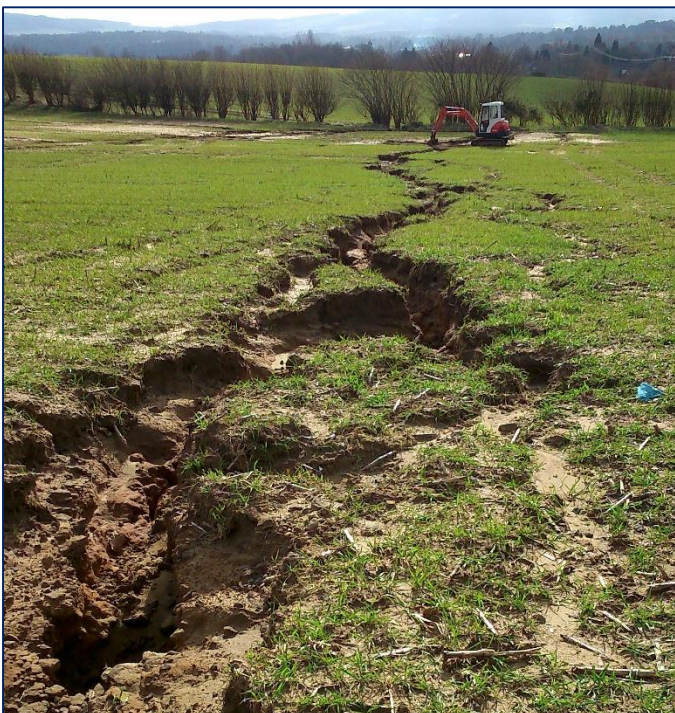
Soil erosion on the fields above Easebourne
