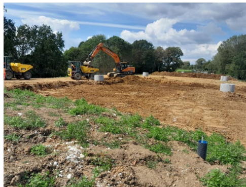
Image 1: Material being removed from the front of the surcharged to be placed further back.
