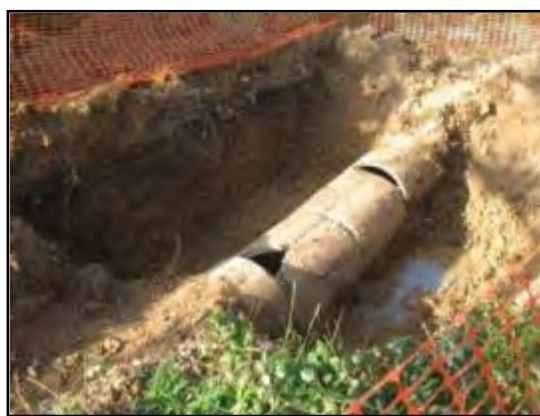
A damaged culvert requiring repair
