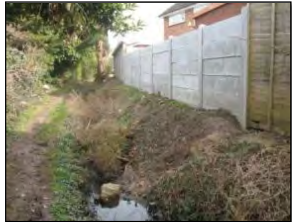
A riparian ditch in need of maintenance to remove vegetation, silt and debris
