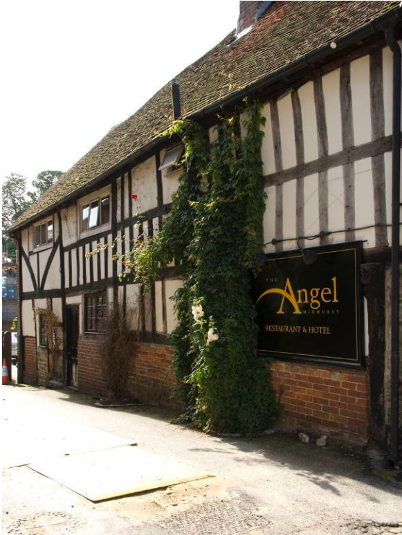
Fig. 15. Tudor View, North Street: side (north) elevation showing 16 th -century timber frame.
