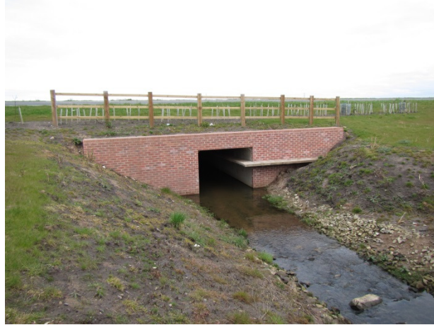
Figure 2- Culvert with Ledges for Mammal Passage
