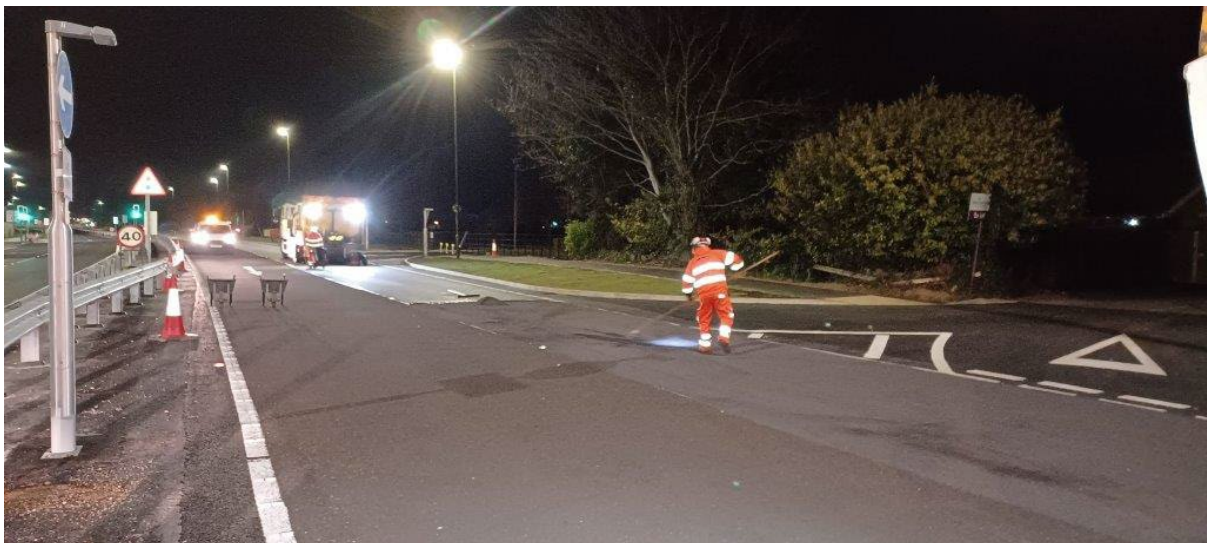
Figure 1: High Friction Surfacing being applied to the new dual carriageway outside Lowertrees on the lead up to the A280 roundabout.
